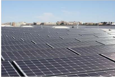
Rooftop Solar Array
