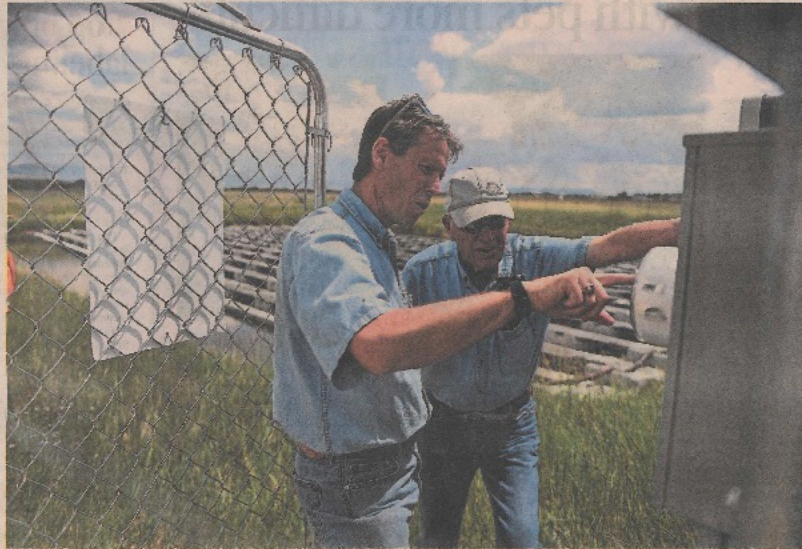
Scott Simmons, left, assistant general manager and engineering manager of Mountain Parks Electric, and Carl Trick, director of Mountain Parks Electric, read the meter of the floating solar array that feeds into the power supply of the Walden water treatment plant on Aug. 22. Alicia Olivares, The Denver Post
